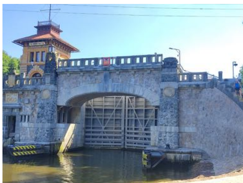
Fig. 3.: The lock of the lock chambre with the Hořín bridge and hydroelectric power plant, part of the Vraňansko – Hořín navigation canal cultural monument. The profile of the lock chamber no longer fits the dimensions of contemporary ship assemblies. The preservation of the structure was achieved by technically demanding widening of the bridge span by 1 m and increasing the underpass height by building a unique hydraulic system to raise one of the spans of the historic bridge by 5 m. (Source: authors)
