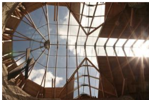
Fig. 6., 7.: Reconstruction of the Church of Neratov, Installation of a Glass Roof, 2006. (Source: )
