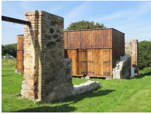
Fig. 2.: The ruins of the barn around the object in Verneřice were partially refilled and stabilised by the authors. (Source: Labor13)
