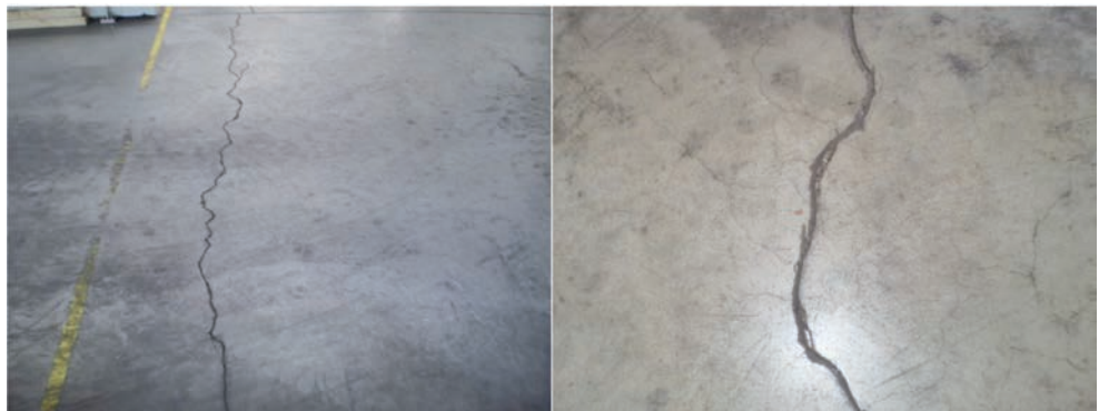
Figure 5 Cracks near the entrance (V1 and V2)
