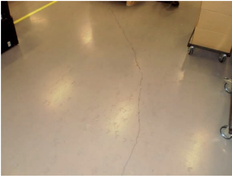
Figure. 10 Cracks on the floor
