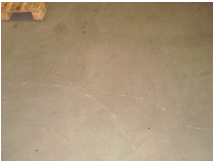
Figure. 11 Cracks on the floor
