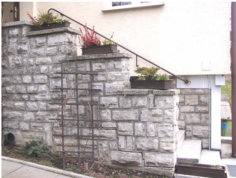
Fig. 5: Damage to the construction of the house
